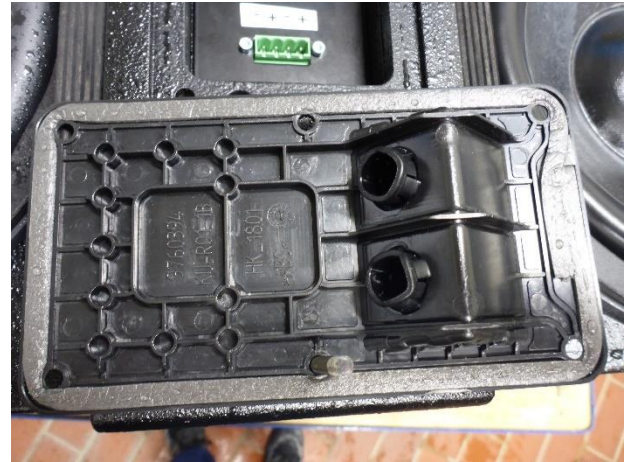
16. Connection Board no ingress of water
