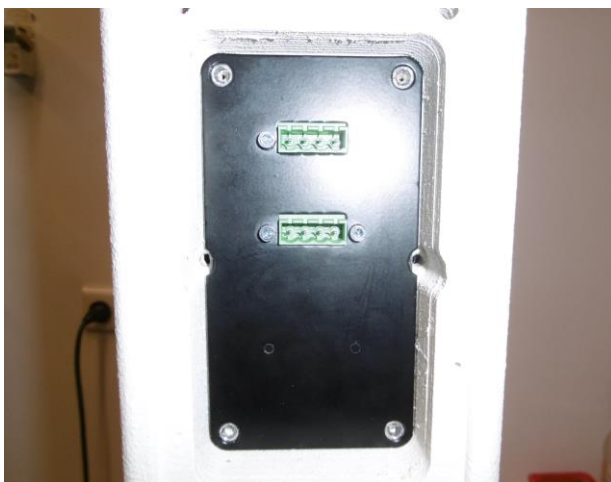
11. Connection box - no penetration of dust visible
