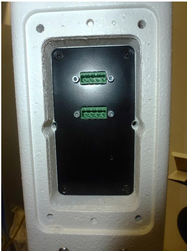
23. Connection box - no penetration of water visible
