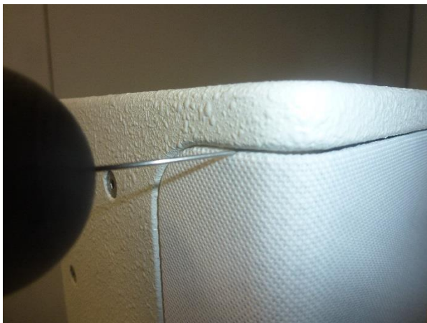
3. Penetration with the access probe \varnothing 1mm not possible
